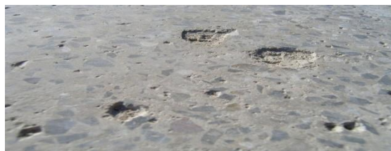
Fig -25: Popouts on Concrete Surface
