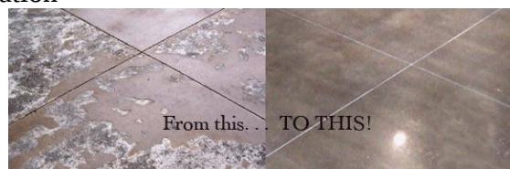
Fig -16: Delamination Before and After Applying Remedies
