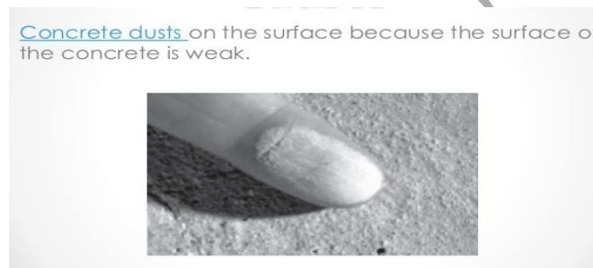
Fig -20: Cause of Concrete Dusting
