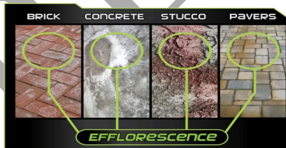
Fig -22: Efflorescence on Brick, Concrete, Stucco, Pavers
