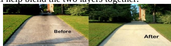
Fig -19: Discoloration Before and After Applying Remedies
