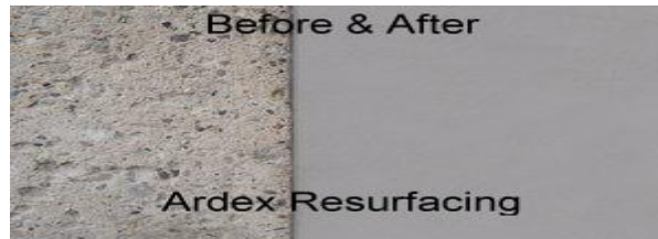
Fig -28: Scaling Before and After Applying Remedies
