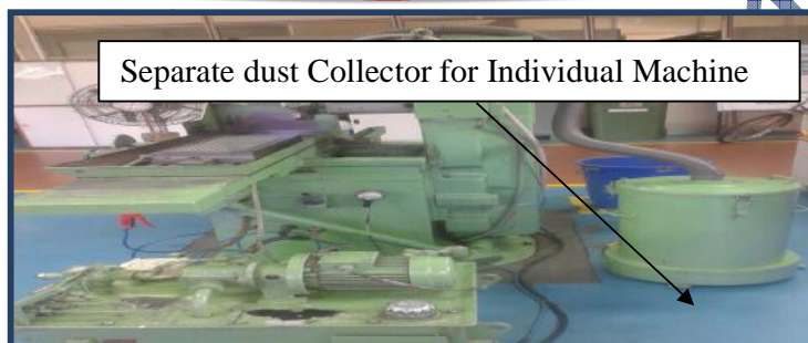
Fig: Grinding machine with separate dust collector. Combined Grinding Dust particle collection system
