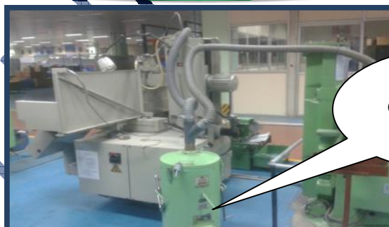
Fig 3.2: Combine dust collector for two grinding machine
