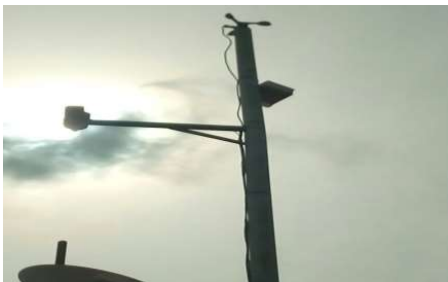
Figure 16: A snapshot of the weather station mounted on a pole.
