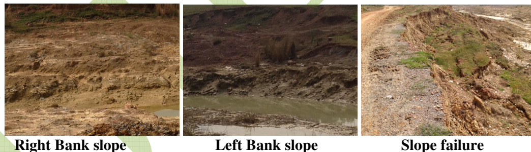
Figure 2 Severely Damaged Slopes
