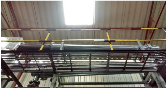
Figure 7: Condenser and Receiver assembly
