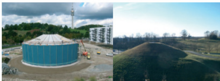
Figure 1 – Large Hot Water Storage (construction and final state) combined with Solar Thermal District Heating “Am Ackermann-bogen” in Munich, Germany
