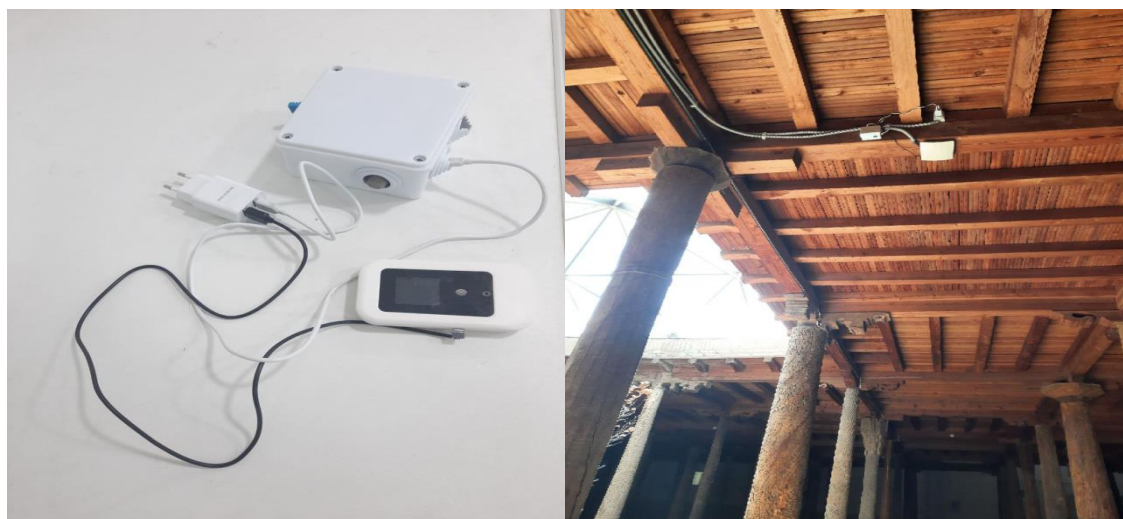
Figure 3. Device installed in Juma Masjid (Juma Masjid)
