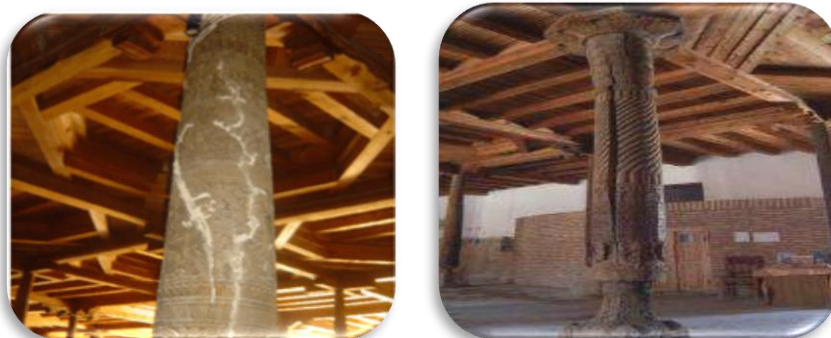
Figure 1. Biological (termite damage) and physical (warping) damage to wooden columns
