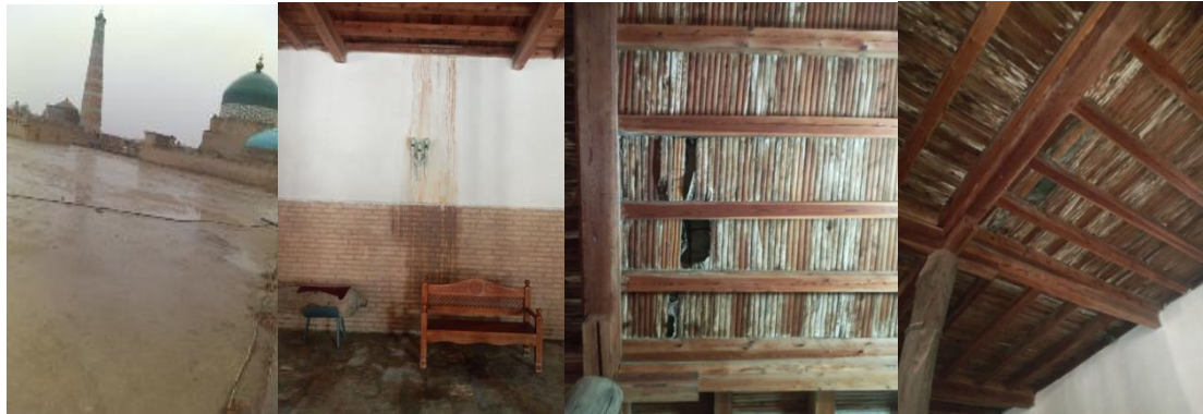
Figure - 2. Rain seeping into the building and damp rotting ceiling
