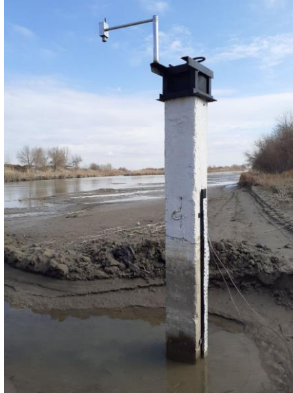
Picture – 1. Smart Water monitoring device.
