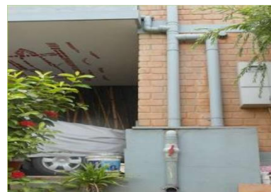
Fig. 15. Provision of Rain Water Harvesting Filter
